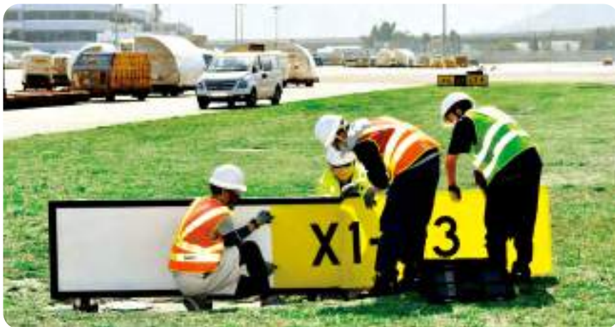
In preparation for HKIA's expansion into a 3RS, the original North Runway, taxi lanes and parking stands are being redesignated.
