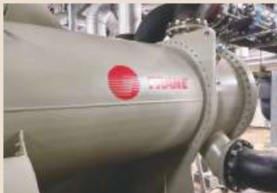
Two 2500TR chillers replaced in FY2022
