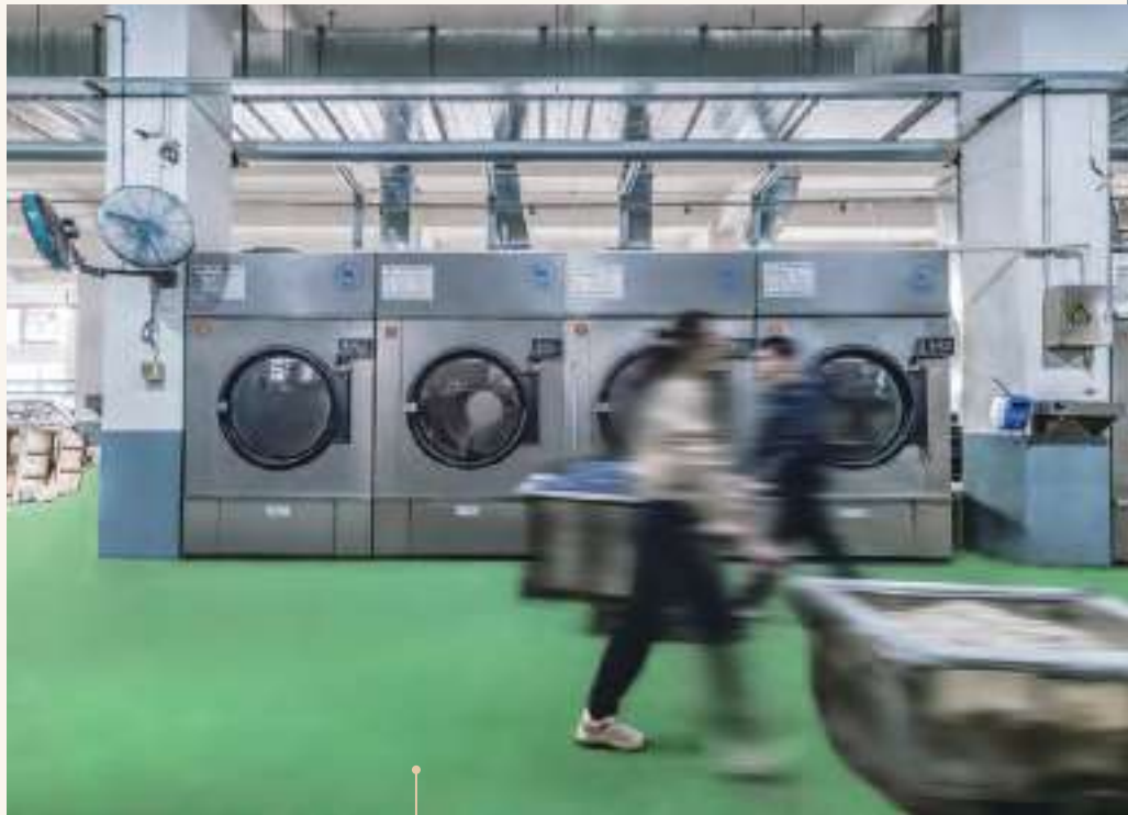
We provide a stable supply of steam to help various clients save energy at the textile industrial park in Suzhou, Jiangsu province.
