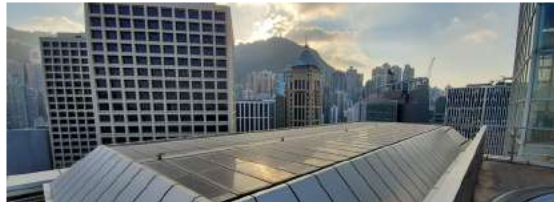
Solar Photovoltaic System at Chater House.
