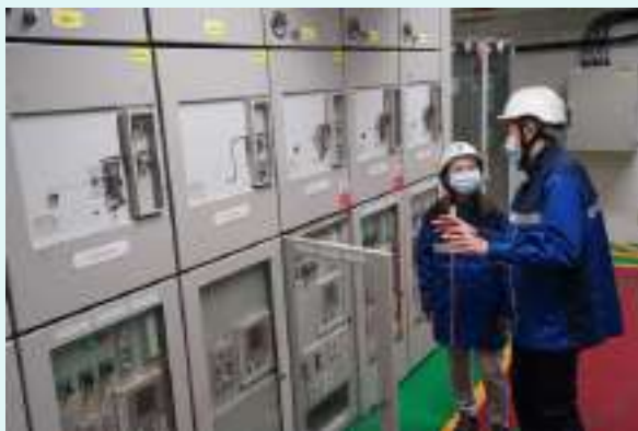
A member of CLP's Graduate Trainee Programme in training to become a power engineer.
