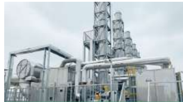
VOC zeolite rotor treatment facilities of Wuxi CR Huajing Microelectronics Company
