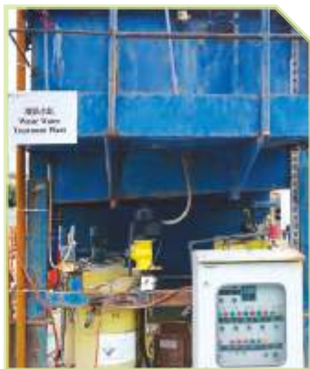
◀ Aerobic Wastewater Treatment System [Anderson Road Quarry R2-2 site] 耗氧污水處理系統(安達臣道石礦場R2-2地盤)
