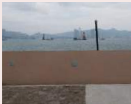
Planter walls at Heng Fa Chuen Playground to prevent the influx of overtopping wave water.
