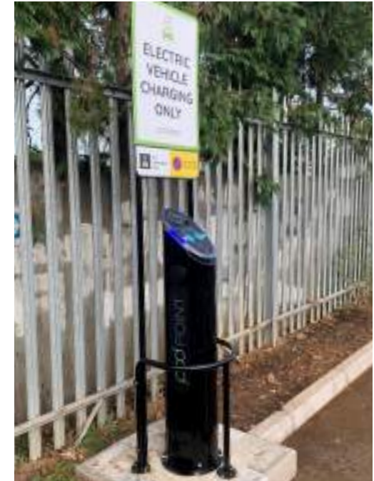
Seven EV charging stations installed at MTR Elizabeth line’s Gidea Park Depot to enable employees to charge their EVs whilst at work.
