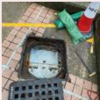
Installation of flap valves at the drainage pipe to avoid back flow of seawater.
