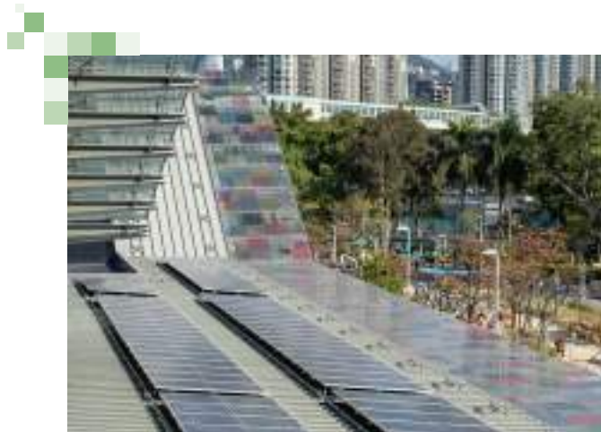
Solar panels installed at roof of Hin Keng Station.
