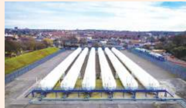
WWU storage tubes for renewable gas
