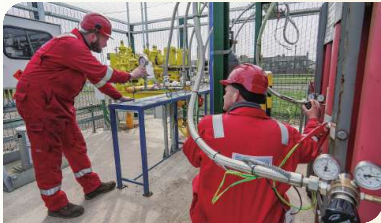
Engineers test operational gas procedures under hydrogen conditions at H21 South Bank site in Middlesbrough.
