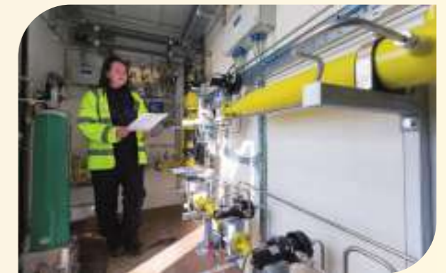
WWU employee inspects biomethane site connection, which supplies renewable gas for the network.
