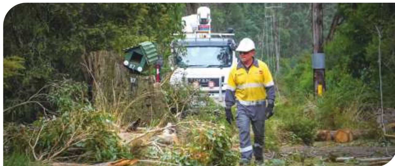
Following a severe storm, VPN crew toil through seriously damaged area to resume customers' power supply.
