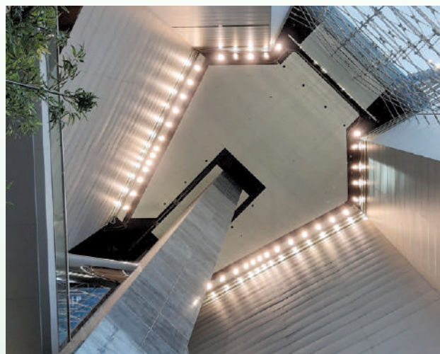
We retrofitted the LED lights with lower wattage ones at the atrium of Three Garden Road to drive energy efficiency
