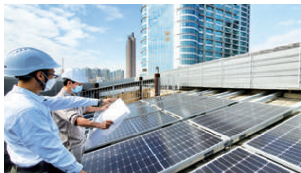
Additional solar panels were installed at both properties in 2022 to leverage sunlight for more renewable energy.
