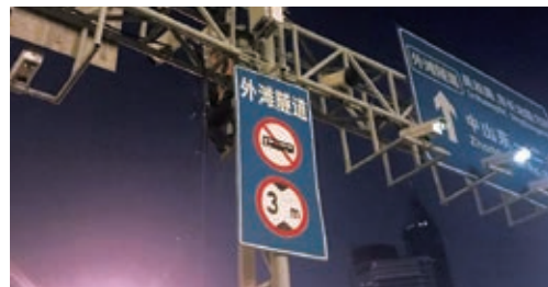
▲ Simultaneously completing 4G+5G coverage by using urban overpass – gantry
