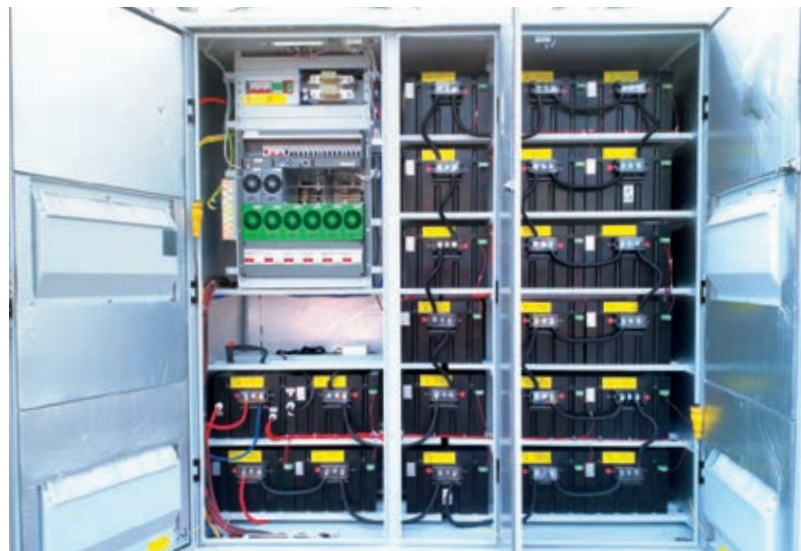
▲ Application of lithium titanate battery
