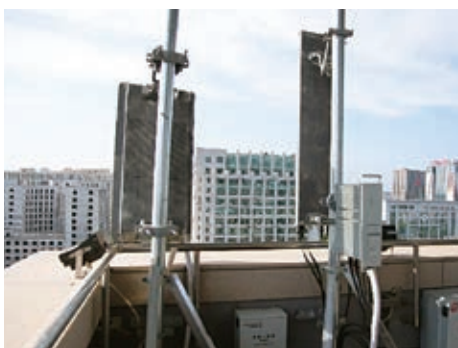
▲ Deployment of 5G facilities on the rooftop of Henan government
