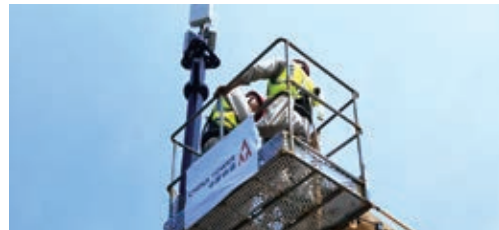
▲ Improving 5G coverage in core areas by using city integrating local poles
