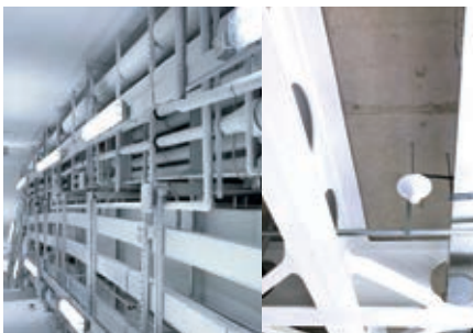
▲ Distributed antenna inside the building
