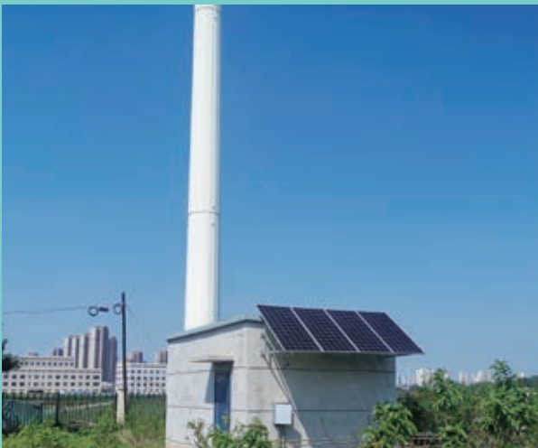
Tianjin Jizhou Stacked Light Base Station
