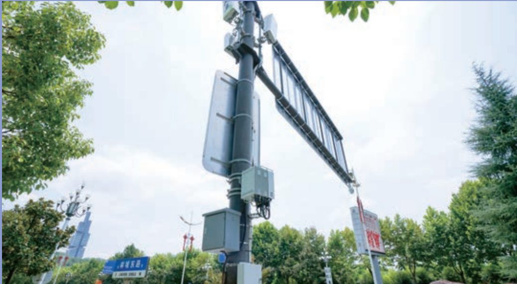
Site for application of outdoor integrated power supply
