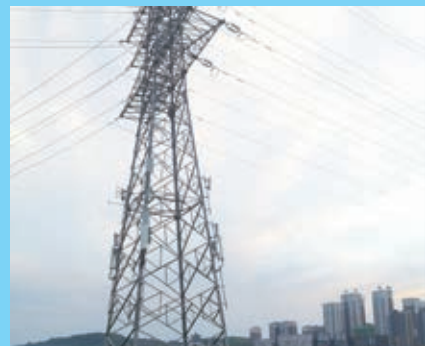
Sharing power tower to solve difficulty in location selection of relocation areas
