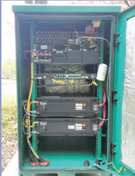
Site for application of modular power supply
