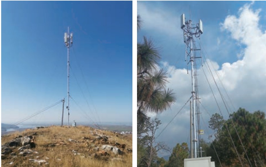
Example of low-cost guyed mast application
