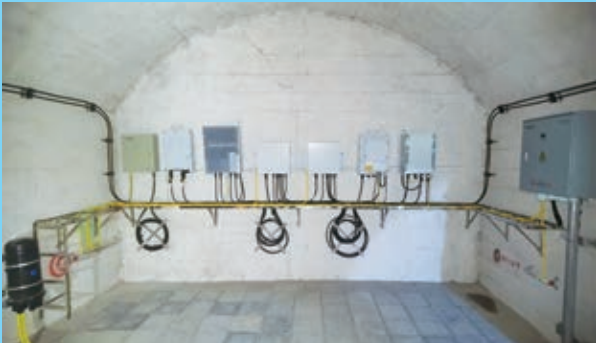
Sharing railway tunnel cabinets
