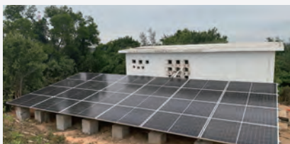
▲ Solar panel and machine room
