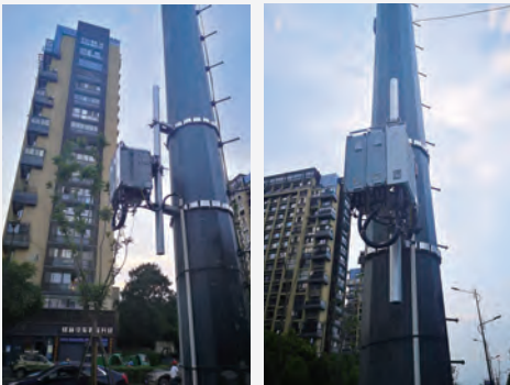
▲ Application of new outdoor power supply in Shanghai
