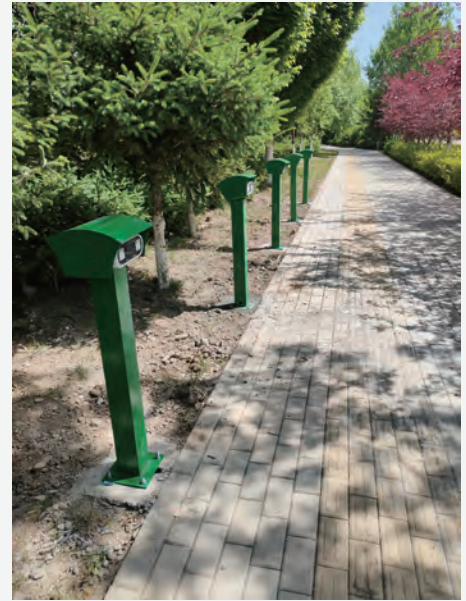
▲ Low-speed electric vehicle charging piles
