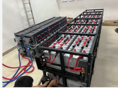
▲ Power backup site of Guangxi telecom communication shelters with power supply facilities supporting
